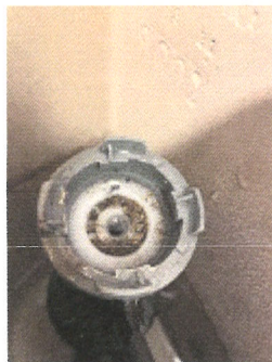
8 Toilet valve plugged with sand..JPG 93K
