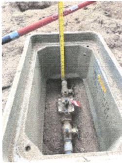
3 Backflow box to shallow.jpeg 182K
