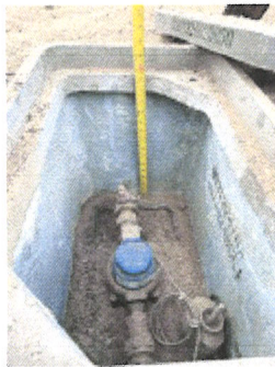
2 Water meter box on uncompact backfill.jpeg 156K
