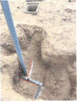
4 wrong size water line.jpeg 124K
